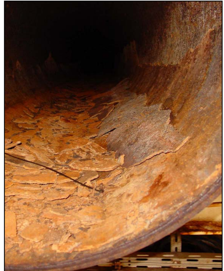
Barium sulphate scale in an oil transport pipe.
